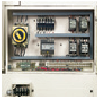
CLEAN, SIMPLE DESIGN AND WELL MARKED ELECTRICS MAKE MAINTENANCE ON THESE LATHES EASY!
